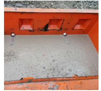
The anchor is cast in its entirety, be careful when vibrating the concrete
